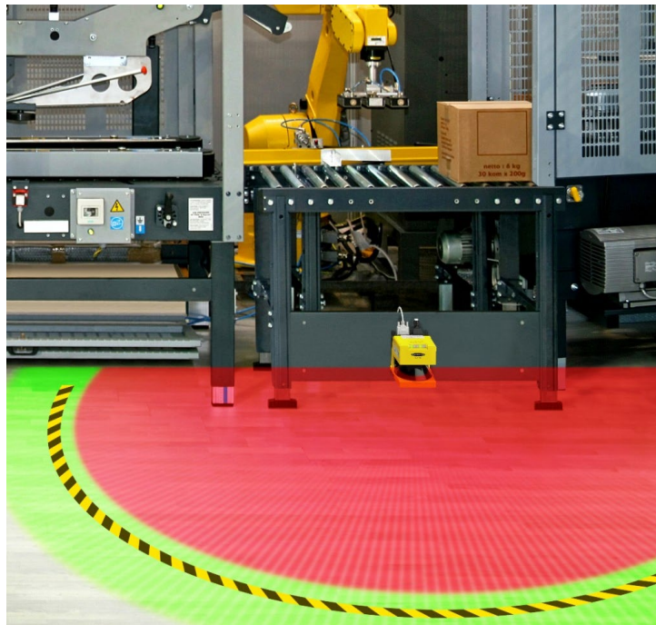
Safety laser scanner provides access protection for robot cell
