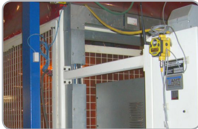
Accurate machine run time data is collected and logged at a control location
